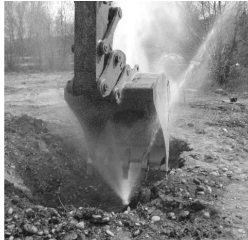
Fig. 2. Consequences of inattentive diggings [3].
